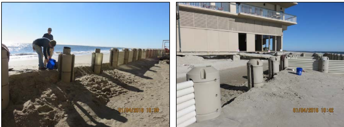
Figure 12: Horizontal panels removed at the Ocean Club WDS in January 2016 to allow sand that was trapped on the seaward side of the structure to continue moving to the landward side of the structure.
