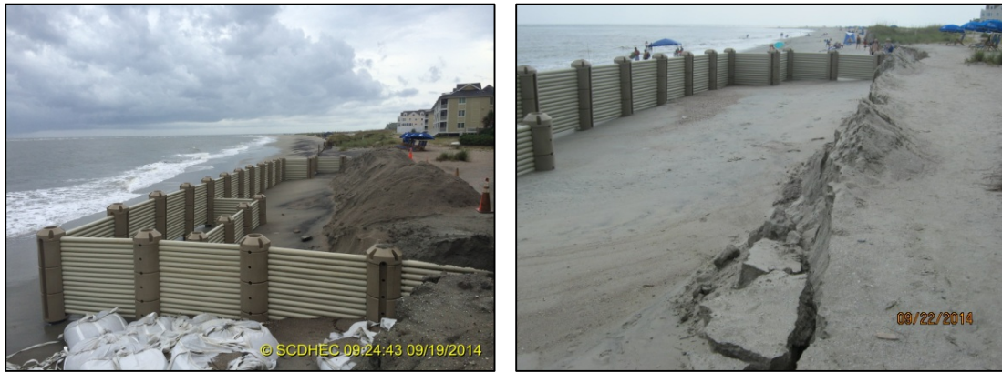
Figure 11: Sand that was scraped and piled up by The Citadel research team at Seascape Villas on September 19, 2014 (left), which had almost completely eroded by September 22, 2014 (right).
