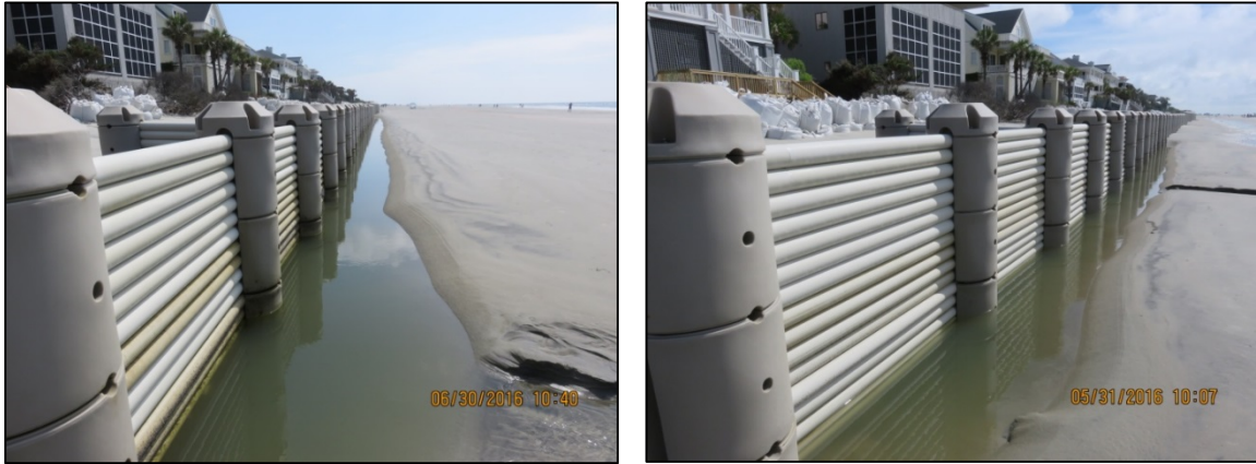
Figure 15: Example of persistent scour (trenching) at the Beachwood East WDS. Similar effects were seen throughout the study at all WDS sites except Seascape Villas.
