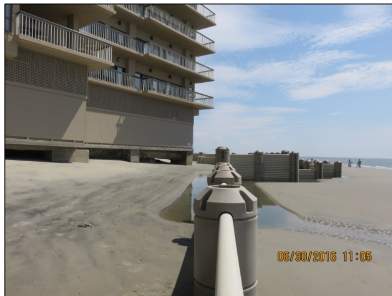
Figure 8: Continued erosion beneath Ocean Club Villas Building #1. Also note the scour (trenching) that is present on both sides of the WDS.
